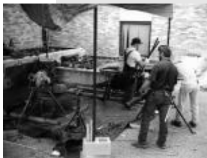
Safety Enhancement Projects - pipe for the Welch Hall sprinkler system is cut and fitted on the south patio.
