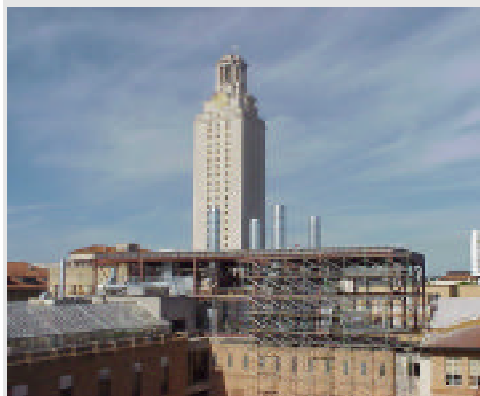
A new air handling system is being installed on the West Wing of Welch Hall.
